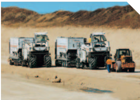
Slurry mixers WM 1000, coupled to Wirtgen recyclers WR 2500 S, producing hydraulically bound base layers.
